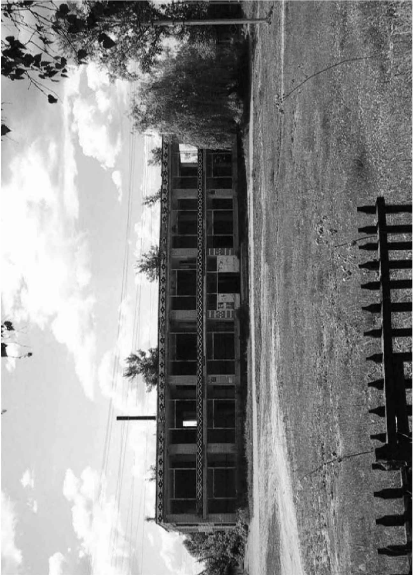
The remnants of the trade centre in Udy, built in the 1970s
