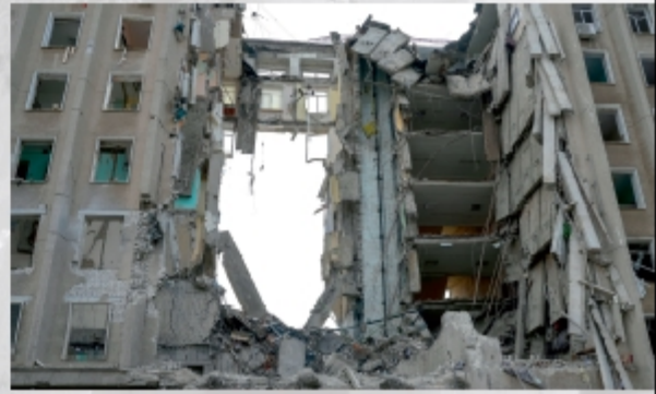
The building of the regional state administration in Mykolaiv destroyed by Russian missiles, March 29, 2022.
